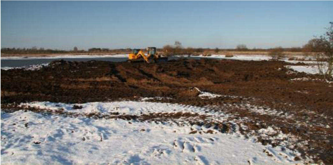
Day 90. Approximately 40,000 cubic metres of soil was taken to the lakes' deposition areas. All material had to be lowered beneath the summer level of the lakes to: (a) adhere to the conditions of the land drainage consent and, (b) to create suitable conditions for the future establishment of reedbeds.
