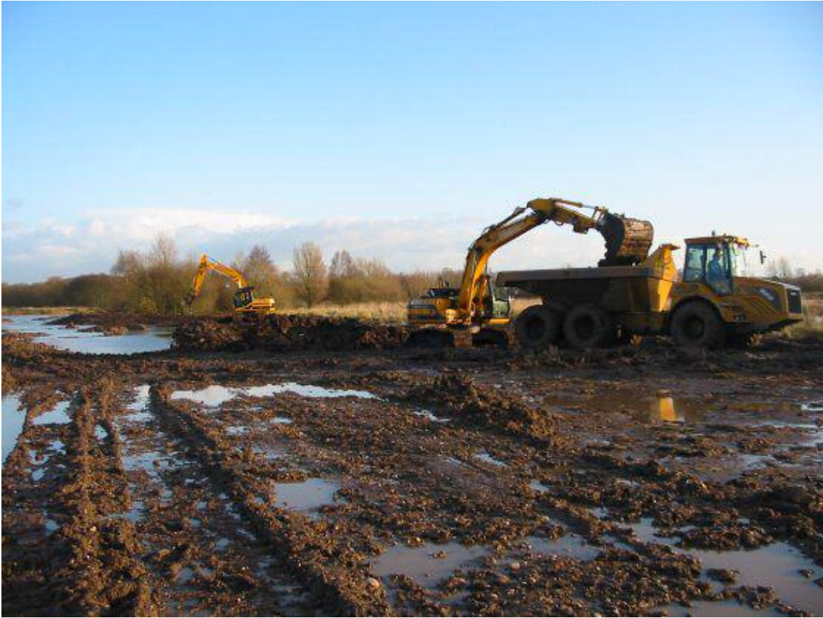
Day 70. Machines with low ground pressure tyres and tracks were used for the scheme to cope with the very wet Autumn and Winter conditions.
