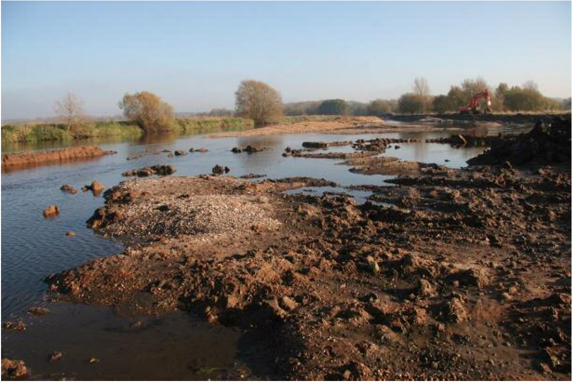
Day 38. Stripping back and lowering at the confluence of the Tame and Trent rivers.
