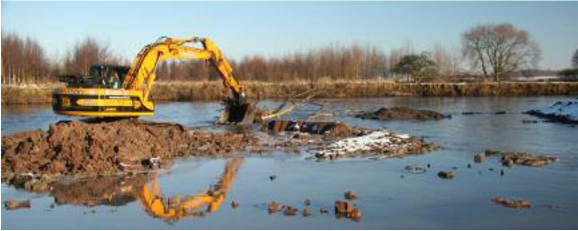
Day 88. Views of river island creation works. Creating scrape in channel substrate.
