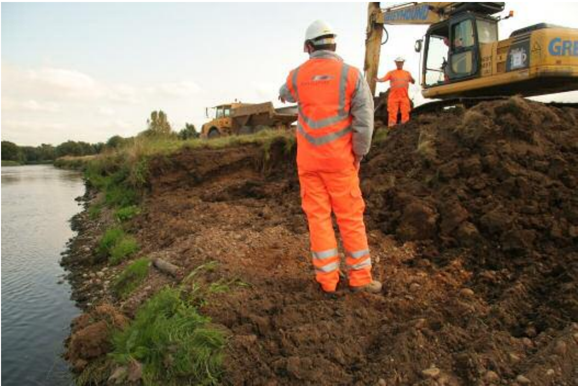
Day 7. Finally! A seam of gravel encountered for the first time and retained for the creation of “braided” channels, mid channel bars, spits and islands.
