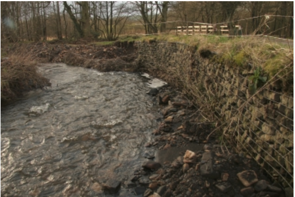
View of the collapsing gabions in 2008
