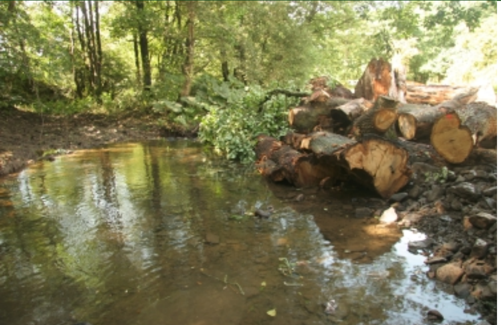
View of the completed ELJ and the entrance to an old side channel.
