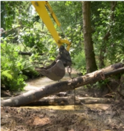
LWD was installed at a number of sites to raise riverbed levels and create additional habitats in the channel.
