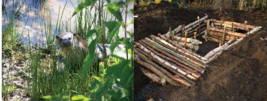
Photos: Otter (left), Derek Crawley/Staffordshire Mammal Group; Otter holt roof under construction (right), Derek Crawley/Staffordshire Mammal Group
